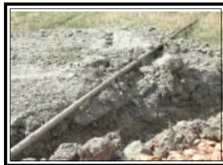
An exposed pipeline near Charlson
